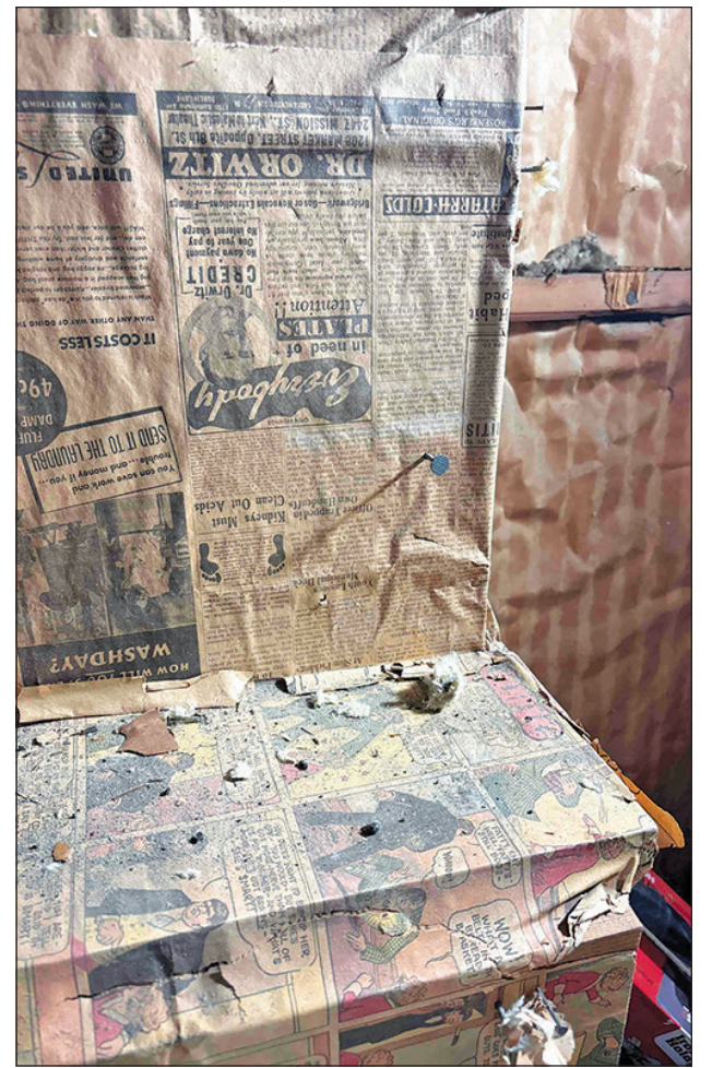
A handyman discovered that a 1937 newspaper was used as insulation in the second-floor addition. Photo courtesy of Andrew Meditz
