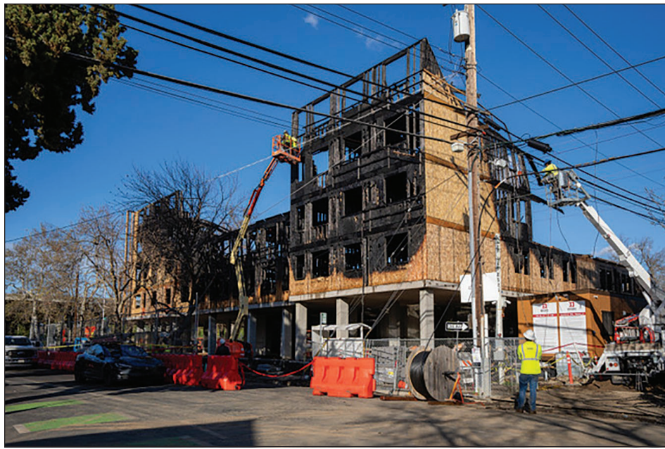
The aftermath of the fire at the On Broadway development site.
